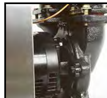
Pump casing bolts
