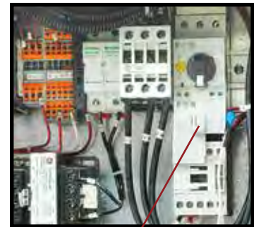
Pump Motor Controller
