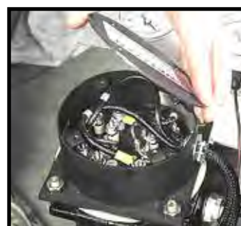
Heater junction wires
