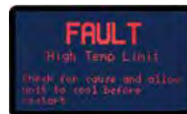
High Temp Limit Fault Screen.
