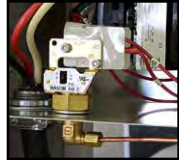
Typical Panel mounted pressure switch
