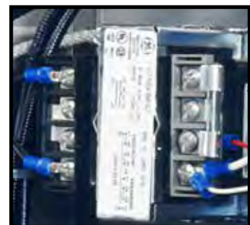
Typical control circuit transformer fuse
