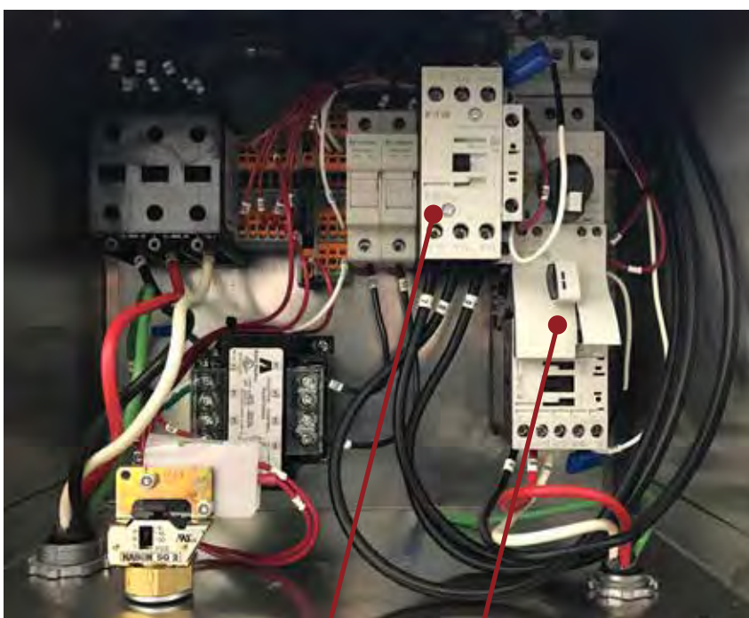
Typical electrical panel.
