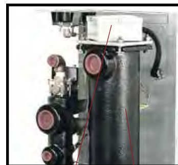
Heater Discharge tank
