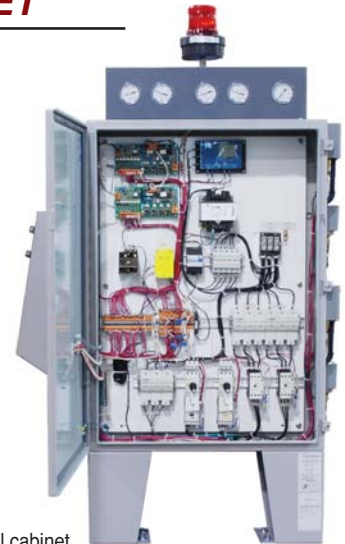
Titan electrical cabinet
