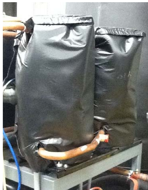
"Deluxe" model compressor sound absorption covers installed on Advantage model TI-80A central chiller with two tandem scroll compressors. Covers provided by Fabricating Services, Inc.
