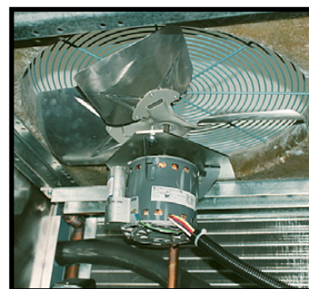
Typical fan assembly
