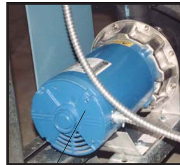
Pump motor Figure 5.5B
