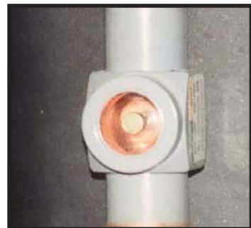
Refrigerant sight glass Figure 6.2E
