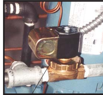
Typical water make-up solenoid valve
