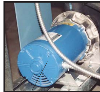
Pump motor Figure 5.5B
