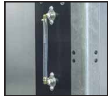
Typical reservoir sight glass
