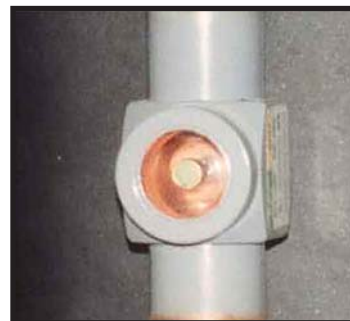
Refrigerant sight glass
